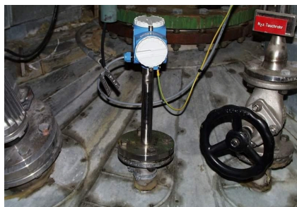
Level sensor installed on a plant vessel
